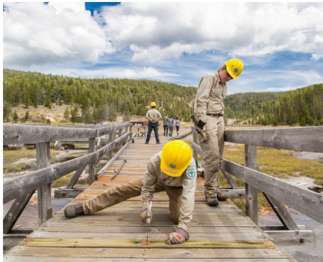
Youth crew members repair a bridge as part of a trail project. Photo by DOI.
